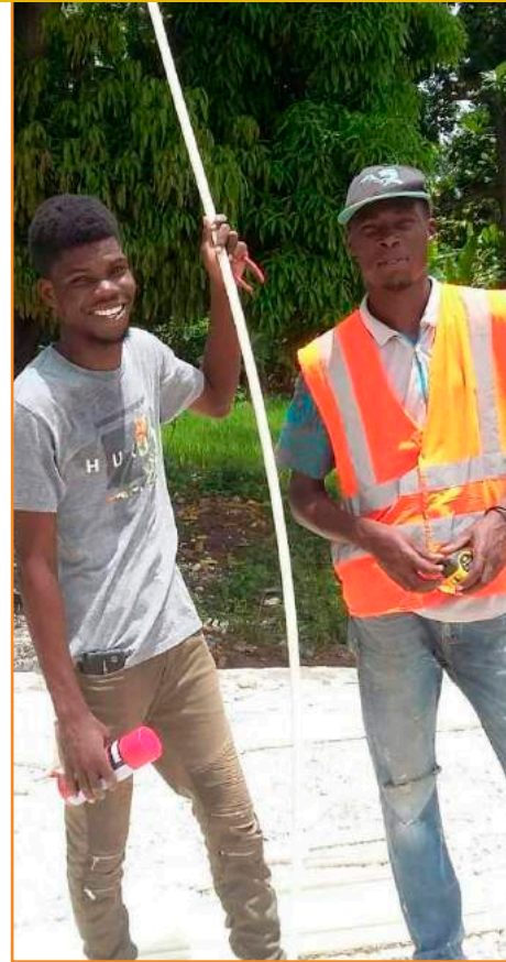
Feguy Francois and Ronsard Raymond at work on a new solar installation in Verrettes.
